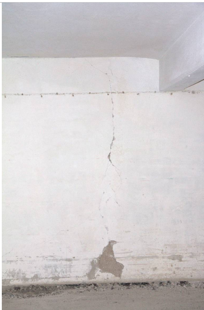
QF_62: quota 7,78 m Fessura verticale
