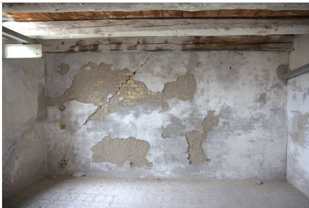
QF_91: quota 10,76 m Fessura diagonale
