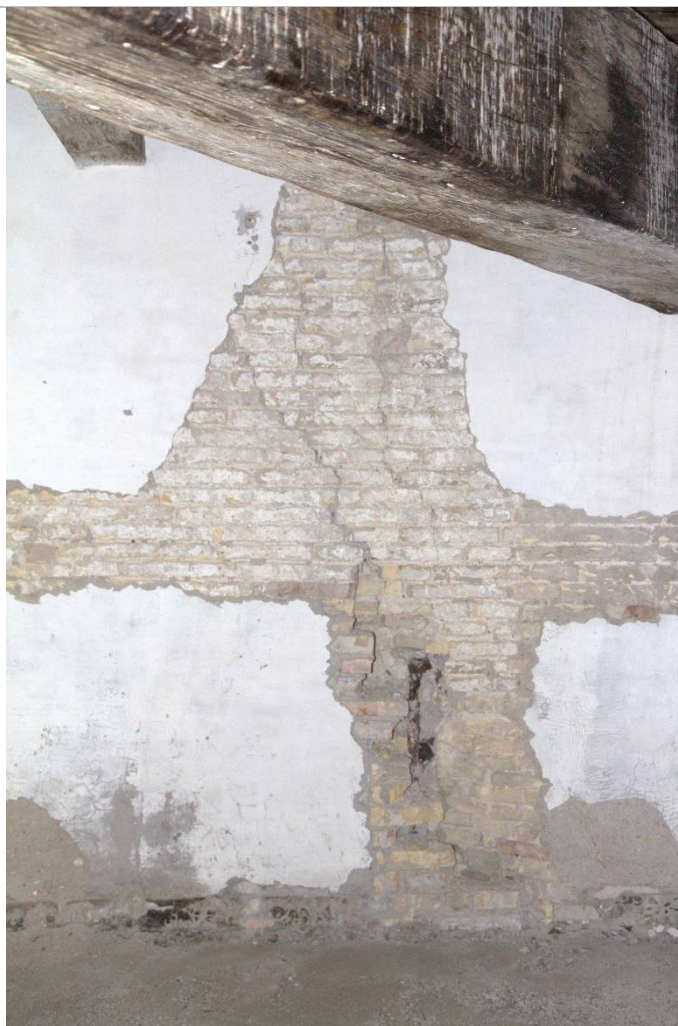
QF_59: quota 7,78 m Fessura verticale
