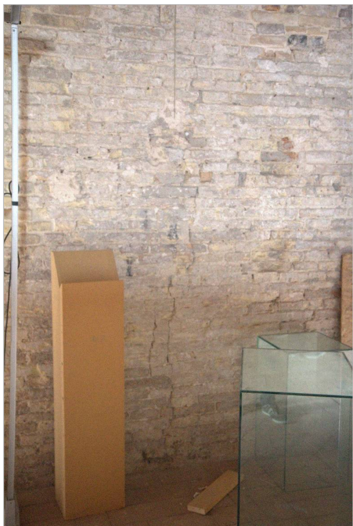
QF_51: quota 7,78 m Fessura verticale
