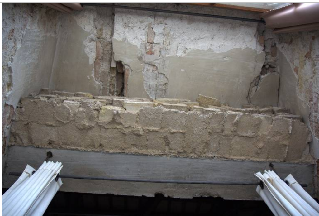
QF_42: quota 7,80 m Architrave mancante
