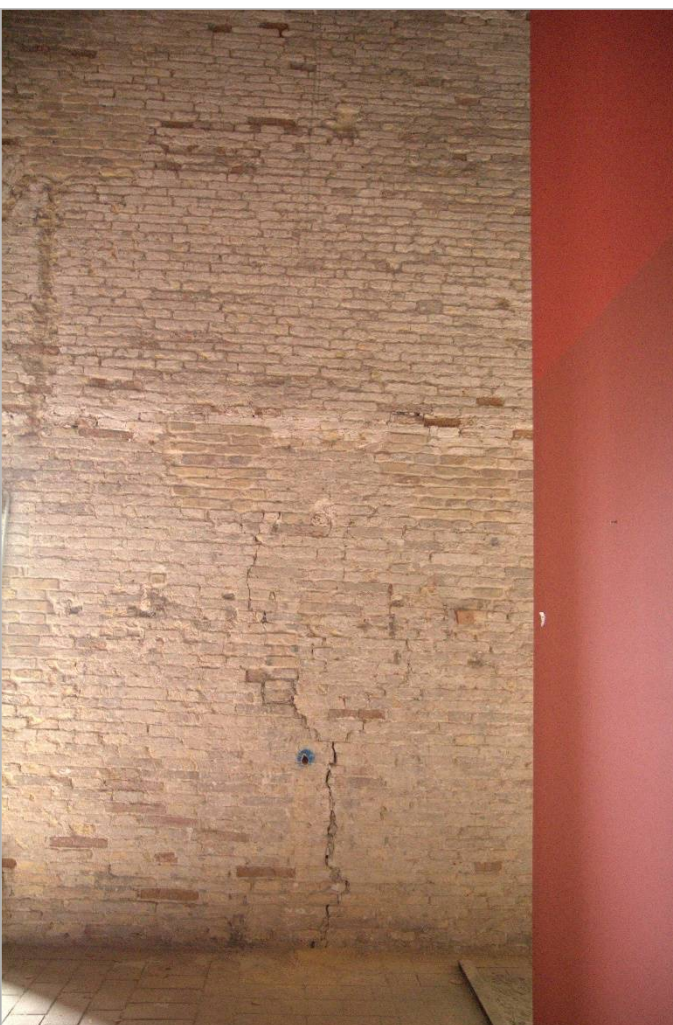
QF_52: quota 7,78 m Fessura verticale
