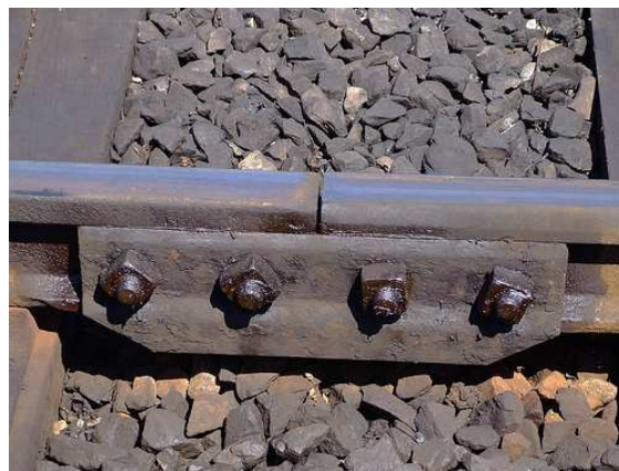
Figure 149. Expansion joint in train rails.
