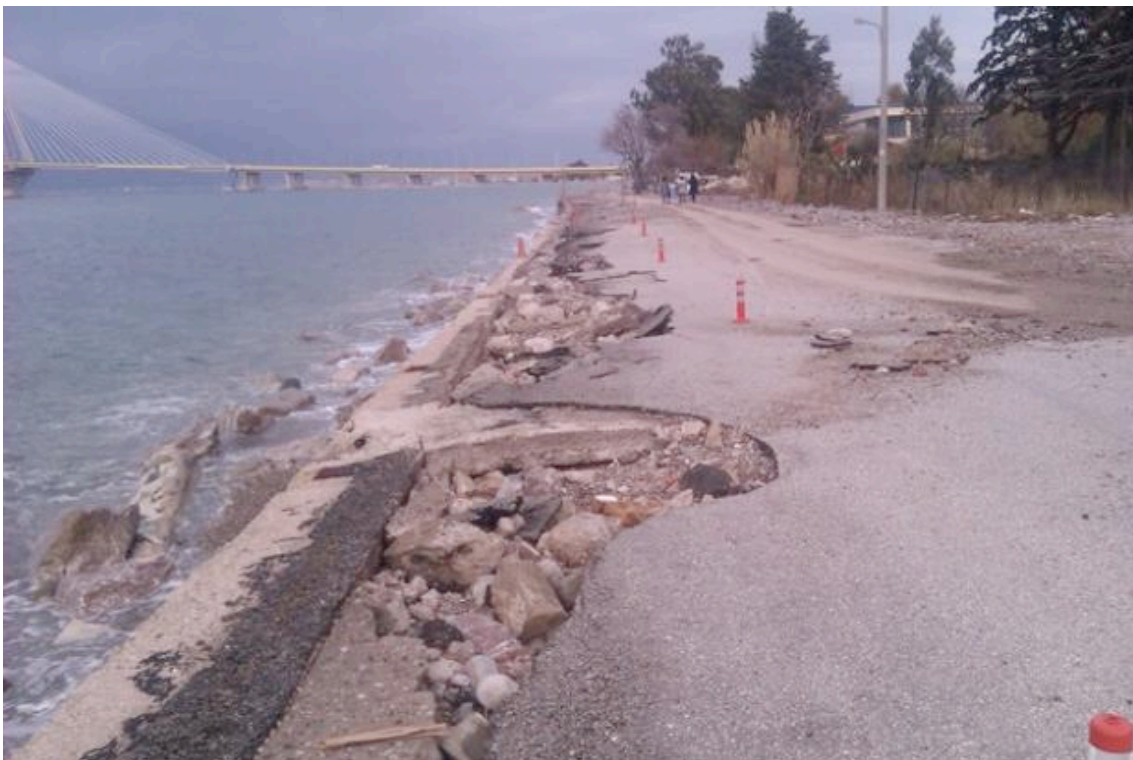
Picture: Coastal erosion in Rio coastline
