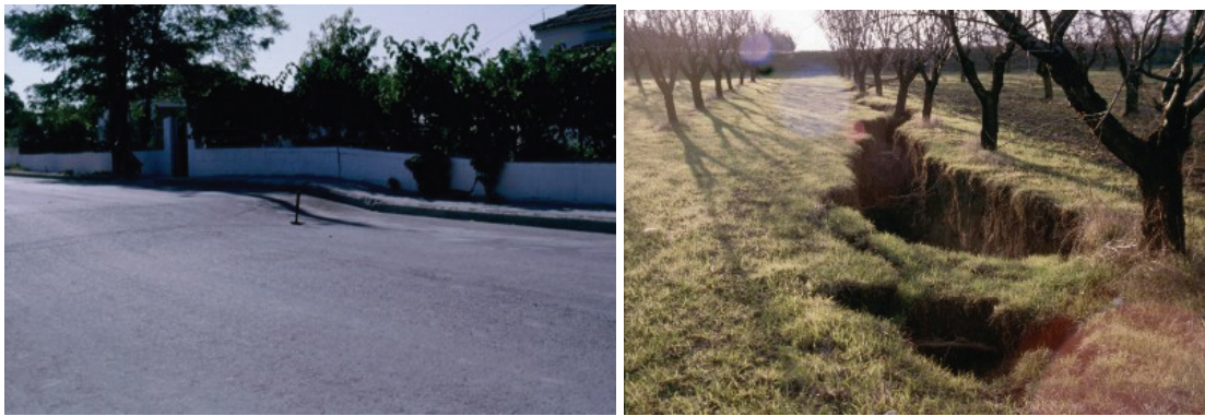
Figure 2 - Left: differential compaction at Nike. Right: ground fissures near Stefanovikio; the 'grass bridge' in the foreground documents the lack of a real superficial lengthening and the occurrence of a piping phenomenon at the surface.
